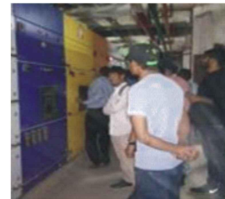
Industrial Visit for students of Civil Engineering to Siddhartha Group an architect excellence, on 20th March 2017
